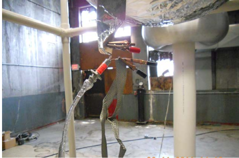
Figure 29. The CVR input and output terminals connect to the strike globe and the ground line respectively. The CVR signal is transmitted on a 25 ft shielded RG62 BNC cable. This configuration was in use while collecting the Table 7 data.
